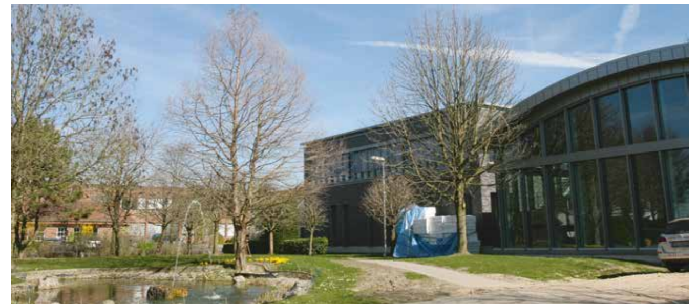
The construction in the Technology Center is progressing according to plan. The building will be opened in early autumn.
